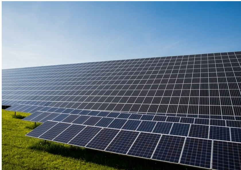
Photo of Canadian Solar panels
